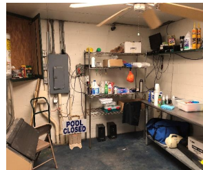
Pool Mechanical Room
